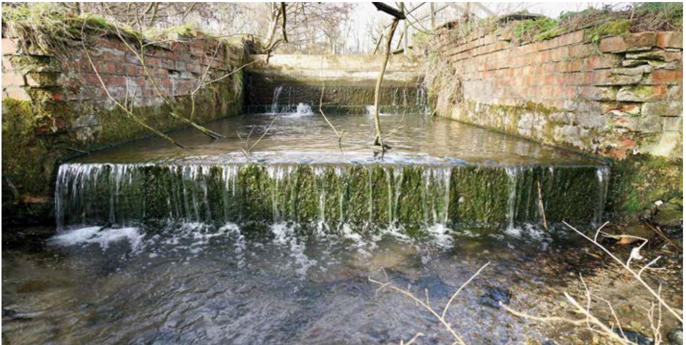
The Shalbourne fish pass before construction. Credits: Rupert Kelton ARK and Cain Bio Engineering
