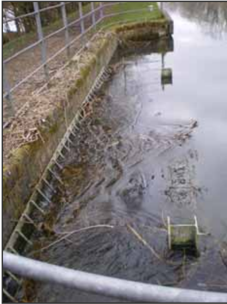
Overflow from canal with screen blocked by debris (perceived poor maintenance). If the screens are not kept clear of debris, the level of the canal rises and the excess water flows over the downstream slipways into the River Dun.
