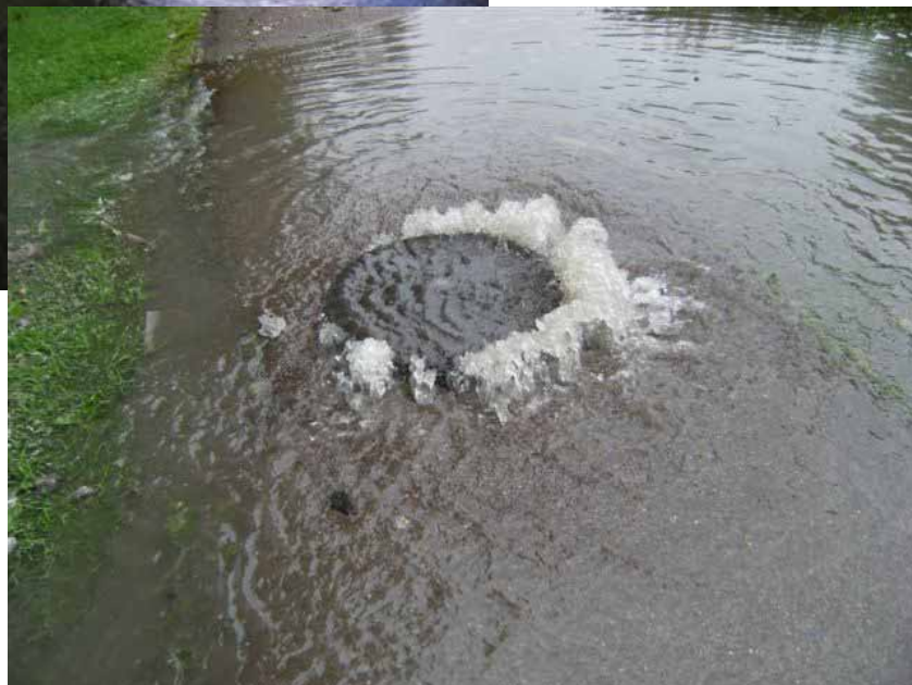
Photo 10 – combined sewer discharge next to the river Kennet at Cooper's meadow Marlborough in wet weather, foul water flowing directly into the river
